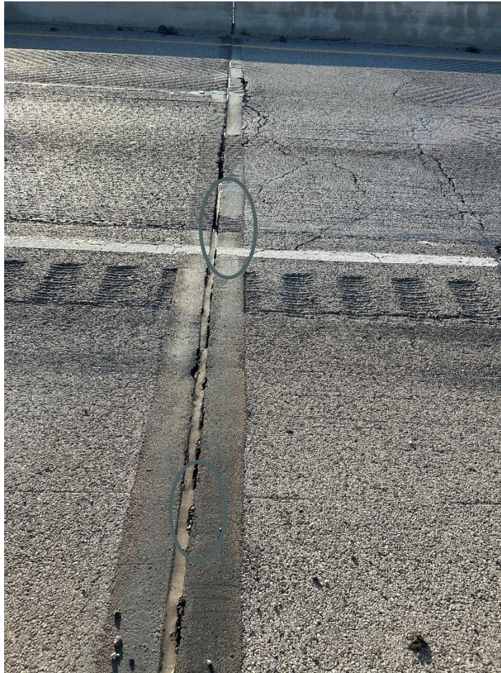
Adhesion Failure – Missing Pourable Joint Material
