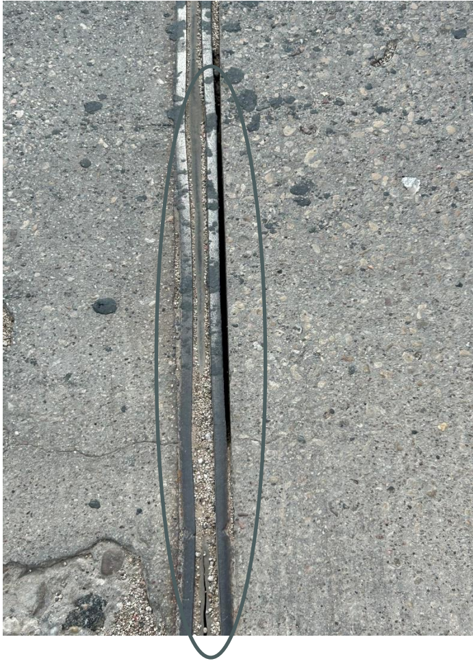
Improper Construction – Expansion Rail Pulled Away
