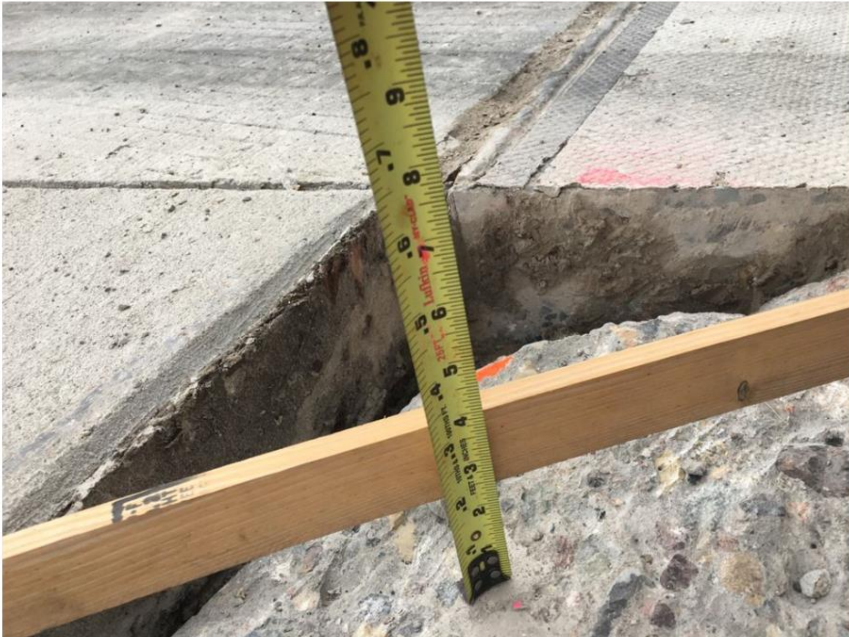
Using a straightedge (lath) to check partial depth repair is a minimum of 2" deep
