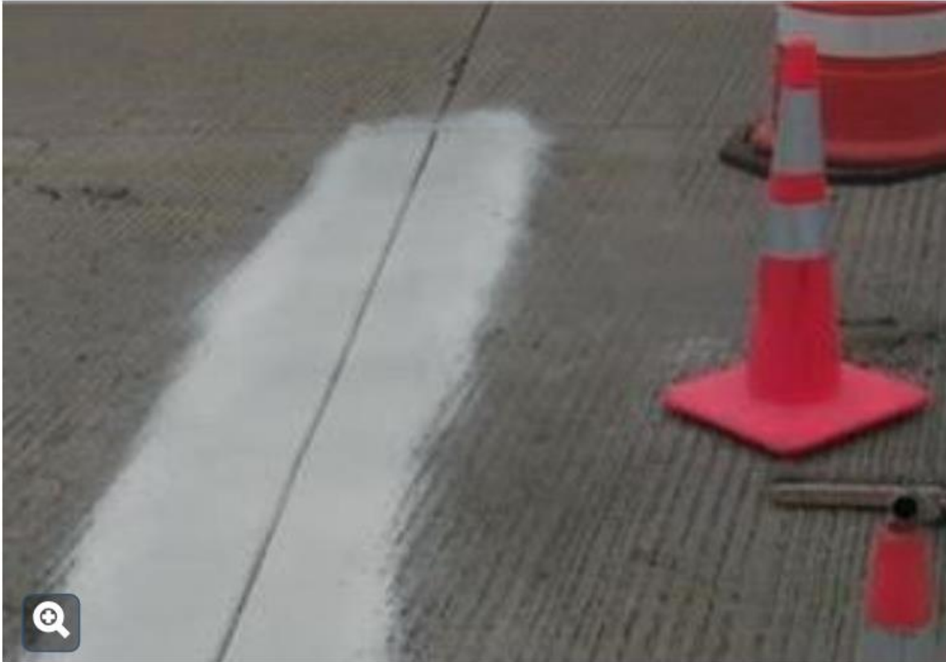
Type B3 repair with curing compound applied uniformly (equal to a white sheet of typing paper)
