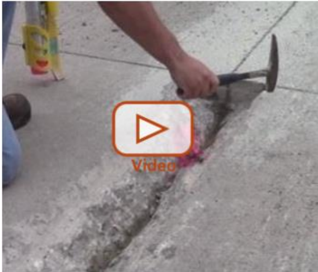
Inspector checking removal area for unsound concrete, misplaced steel, exposed dowel bar ends, and 30° to 60° tapered edges.
