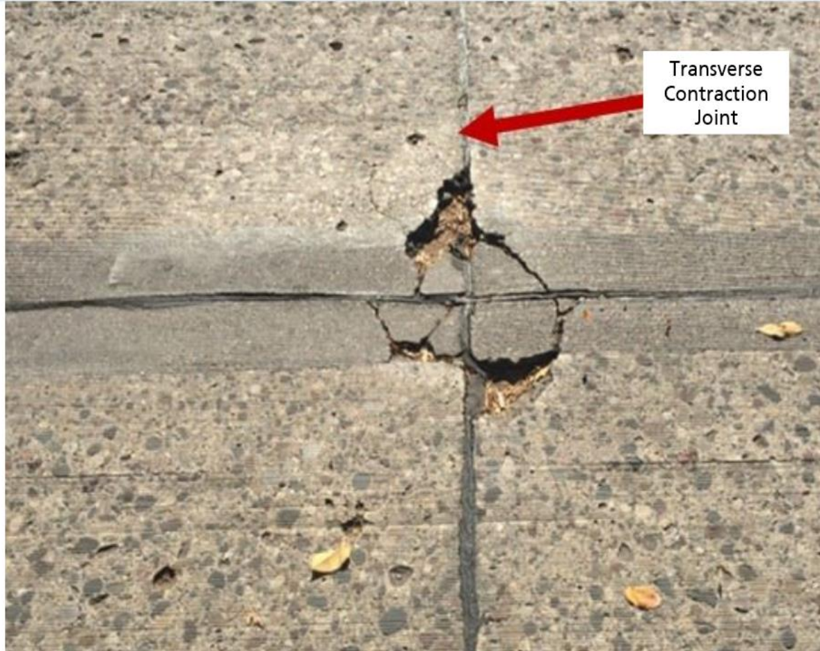
Compression relief not installed at time of construction resulted in compression failure (Picture taken 1 year after installation)
