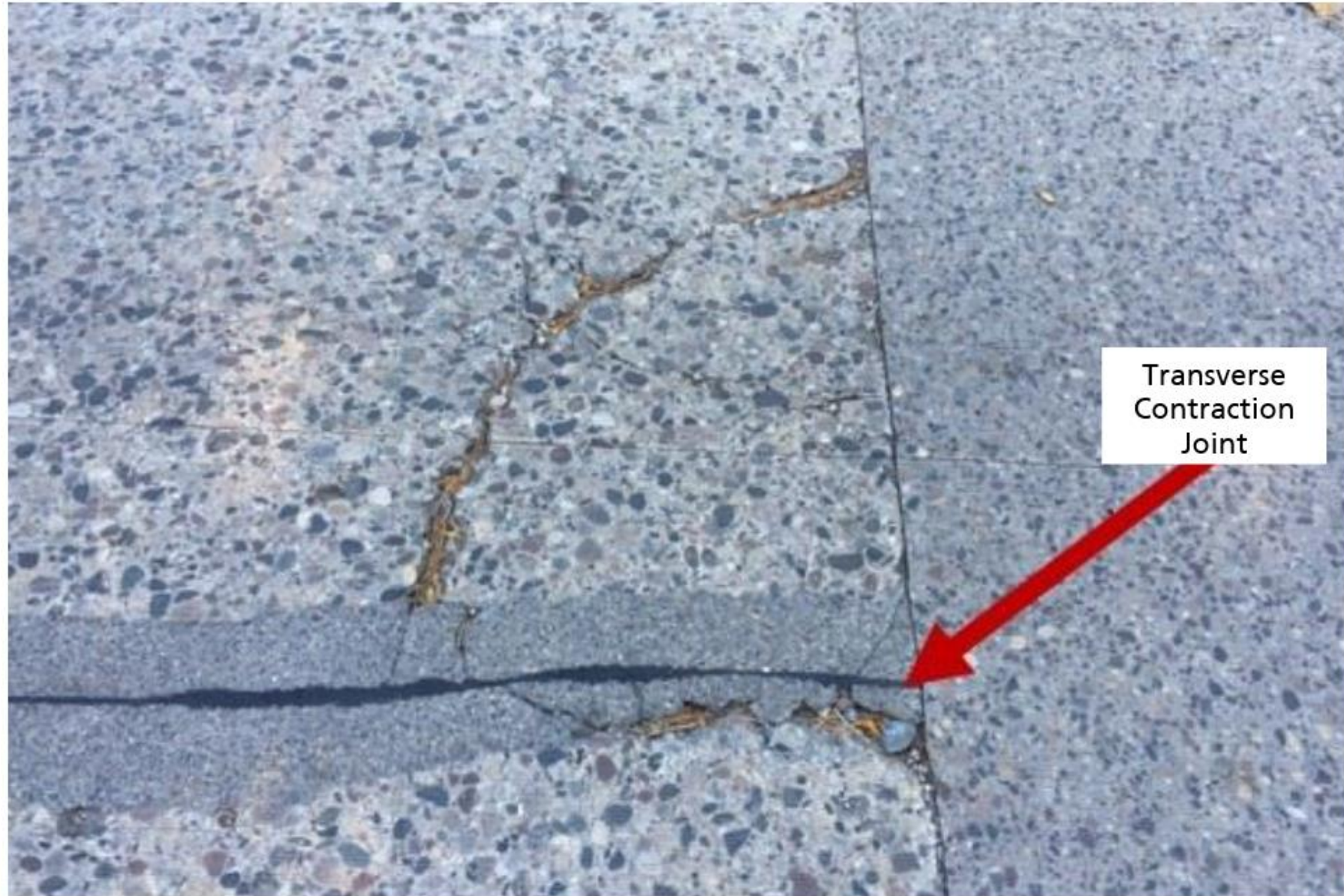
Compression relief not installed at time of construction resulted in compression failure (Picture taken 1 year after installation)
