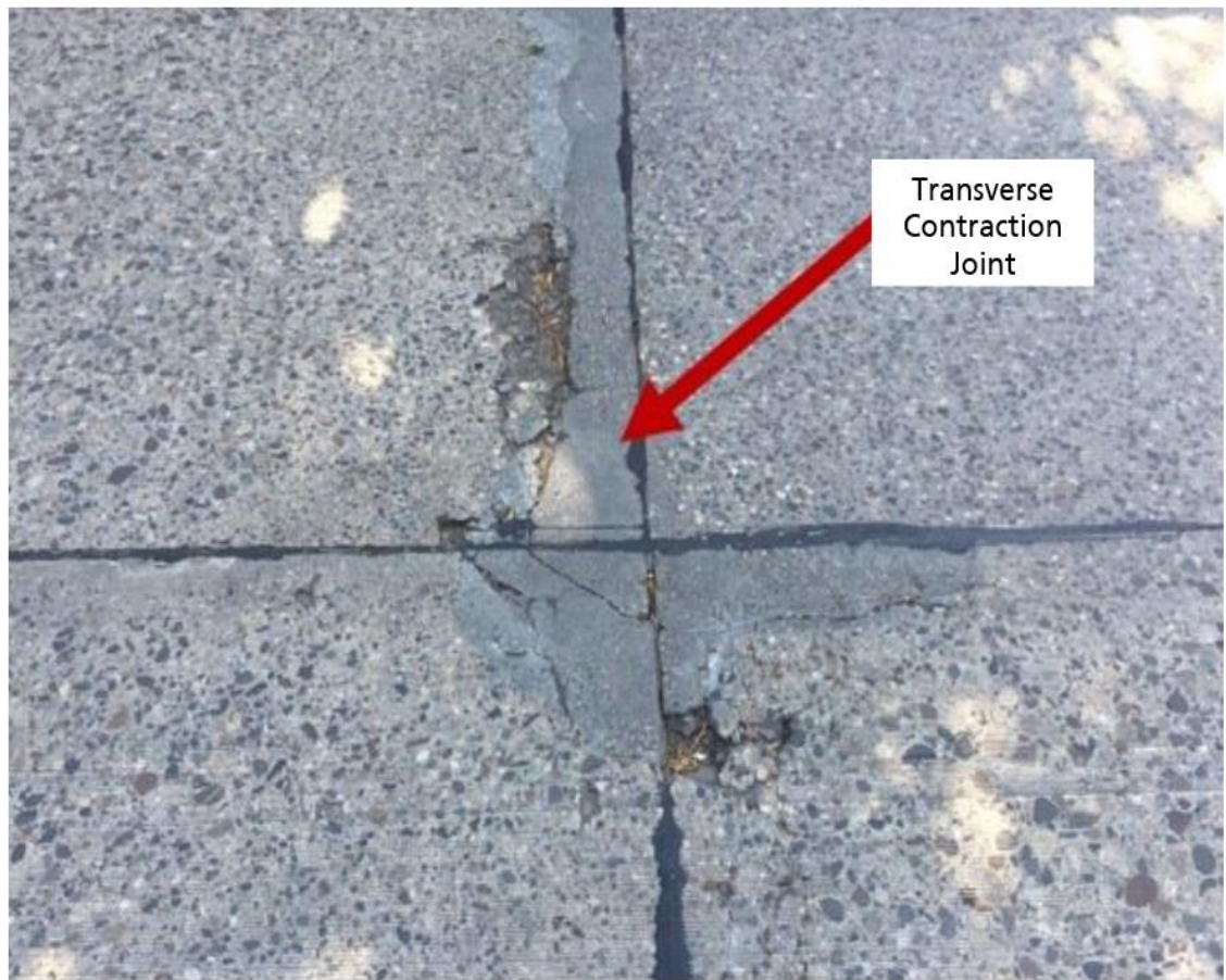
Compression relief not installed at time of construction resulted in compression failure (Picture taken 1 year after installation)
