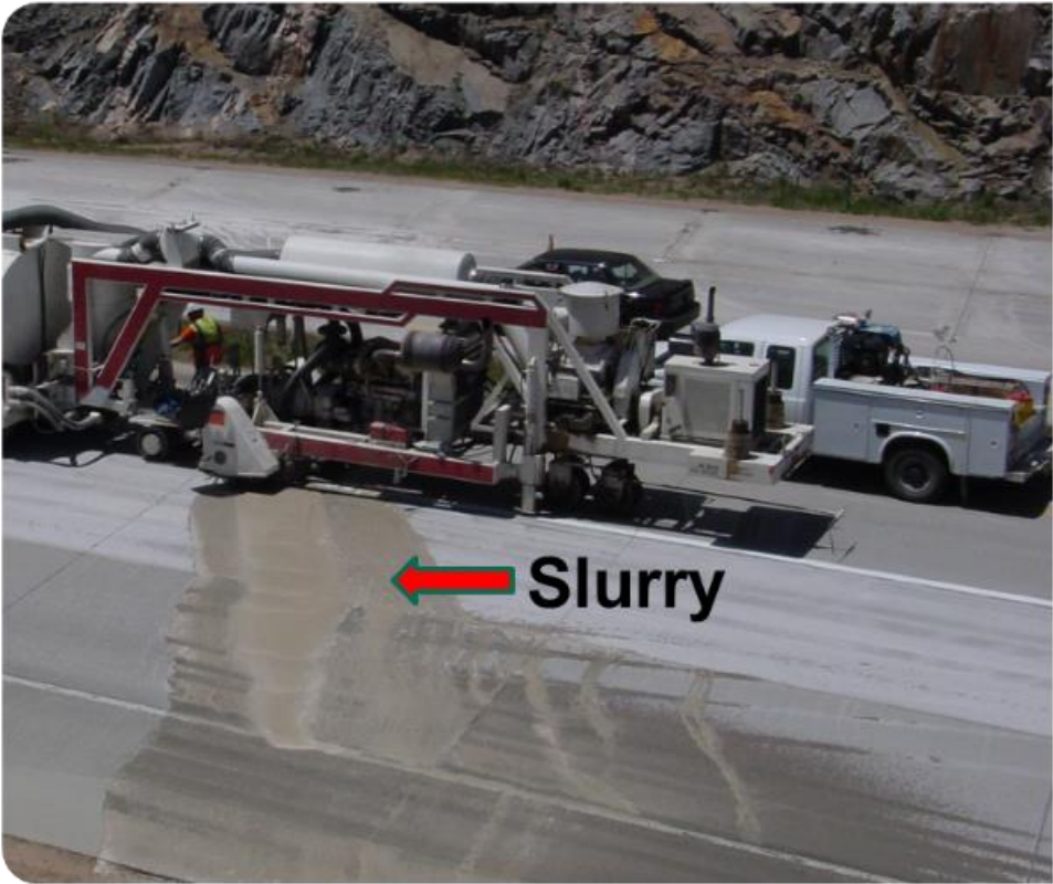
Slurry Recovery Failure
