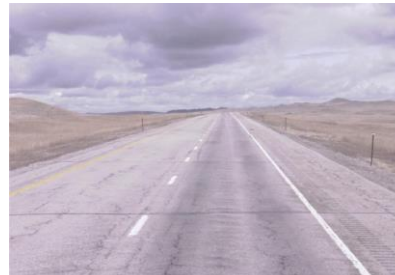
Poor Condition – PQR < 2.5
