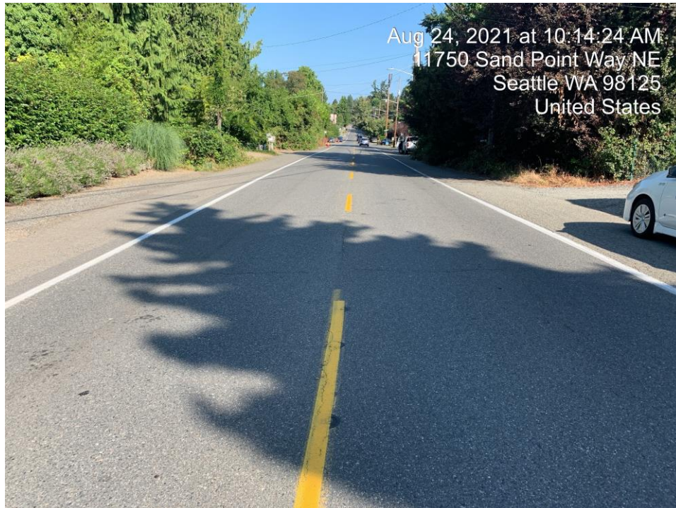
11700blk of Sand Point Way NE - Before crack sealing
