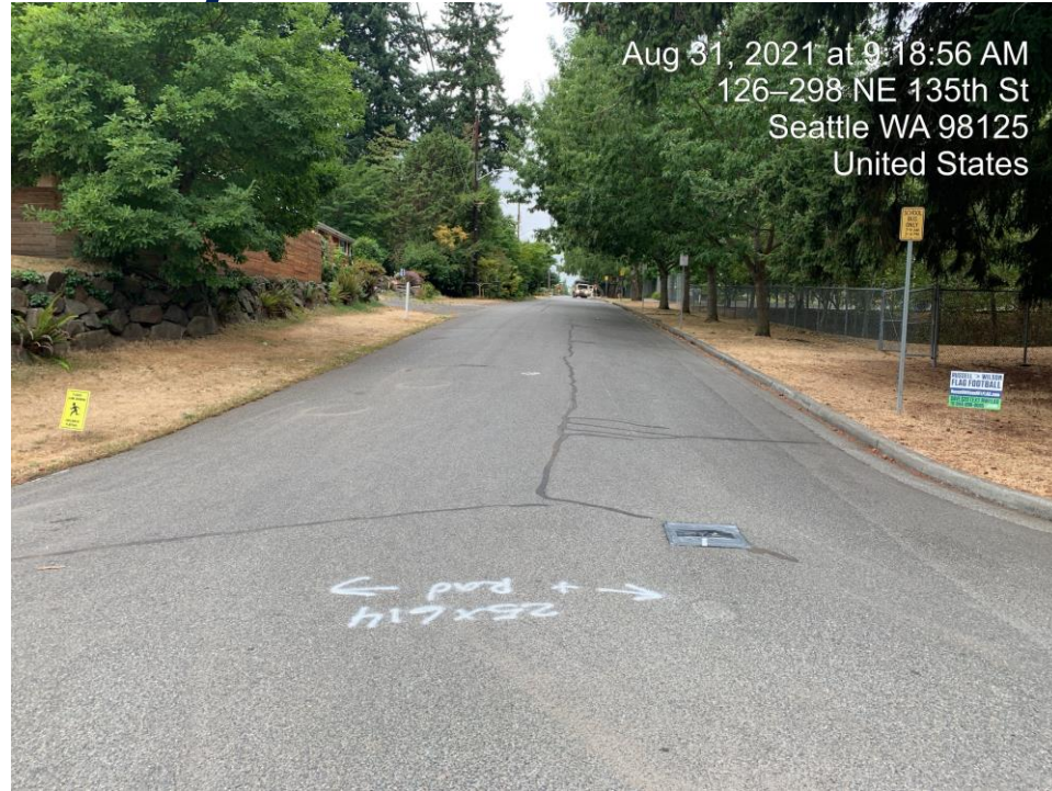
200blk of NE 135 th St - Before Slurry Seal
